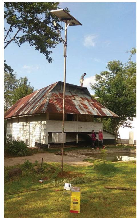
Solar power installed at the TK Wildwood community centre, Paorei, Shirui, Ukhrul.
