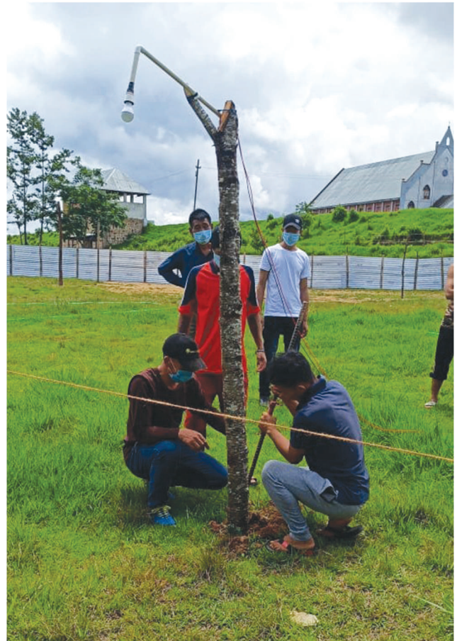
Solar backup installed at community quarantine centre, Ukhrul District.
